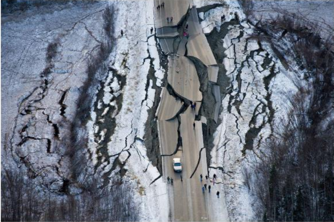
Vine Road, south of Wasilla, was heavily damaged by an earthquake on November 30, 2018. (Marc Lester / ADN)
